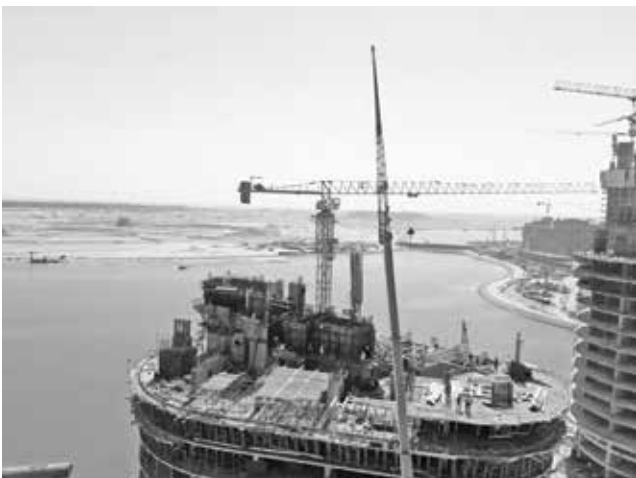
Acrow Board Vertical Walls With Acrow Beam From Basement Up To 28:00 So far, Alamein Towers - Arab Contracting Client
